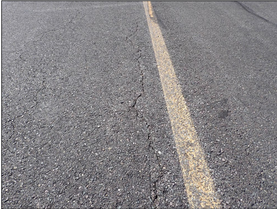
TW-05-03: L&T Cracking
