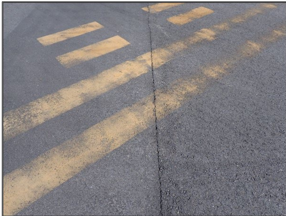
TW-11-01: L&T Cracking
